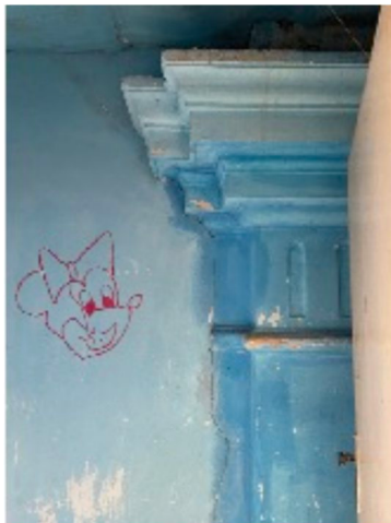
Overpainted decorative elements
