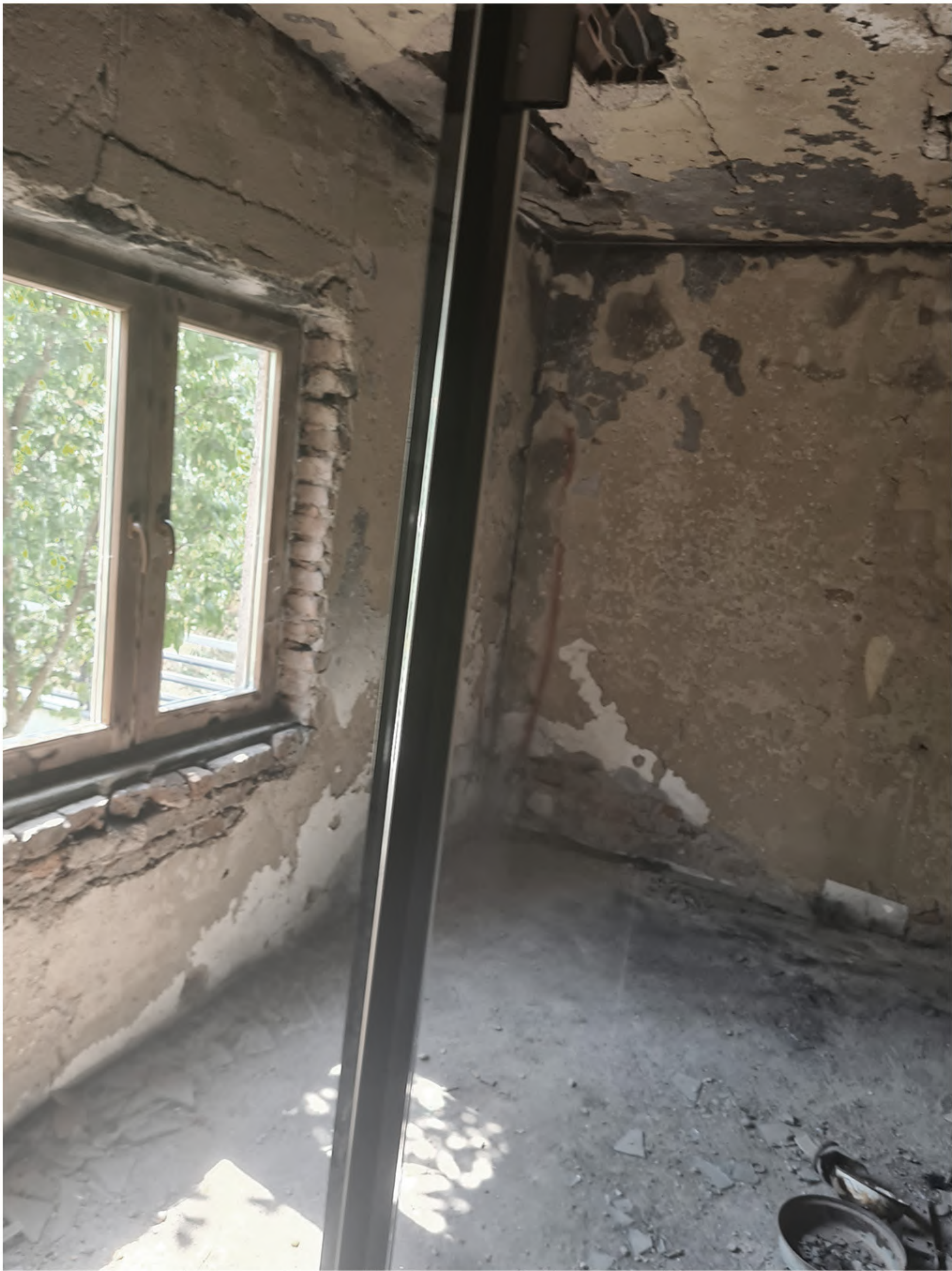
Traces of fire etched in crumbling walls ©project team
