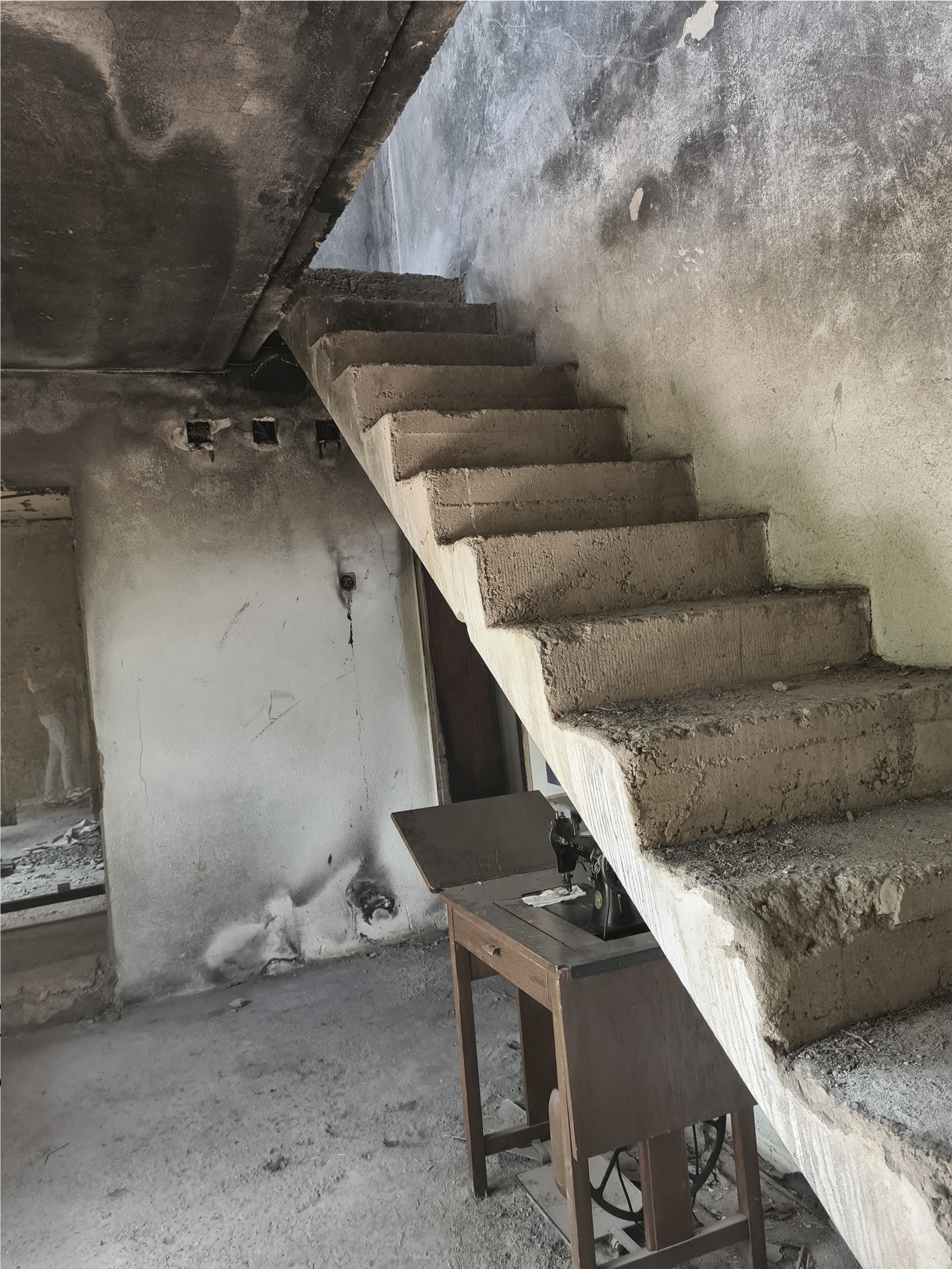
Traces of fire and flight ©project team
