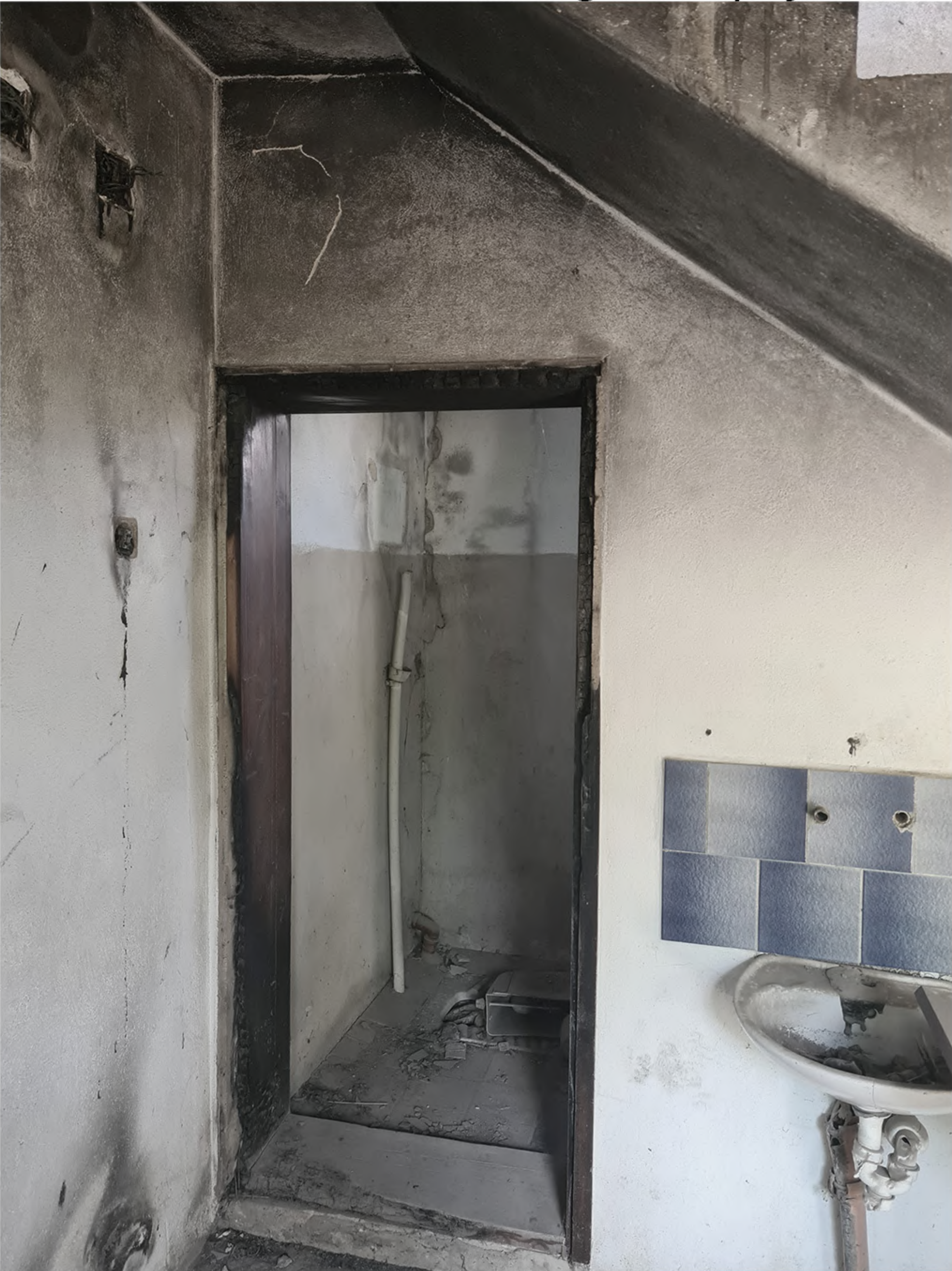
Broken sanitary fixtures—still in place ©project team
